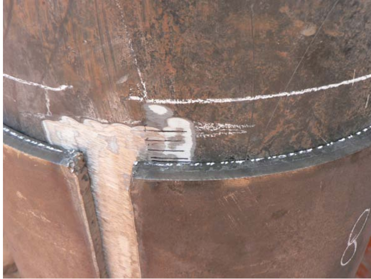
Photo 9 – Amount of displacement on pile sleeve
