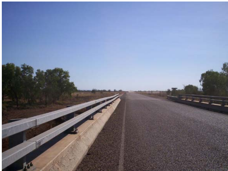
Photo 3 – Deflection in the bridge rail
