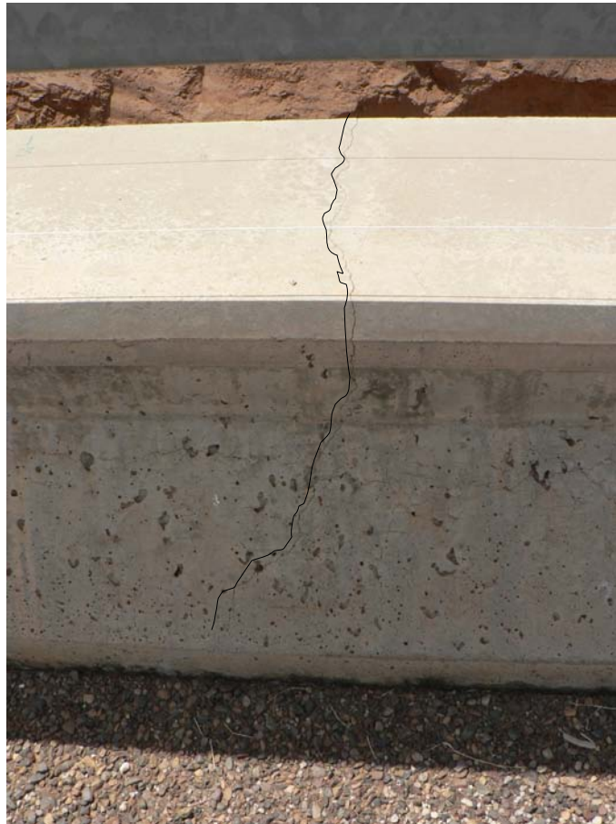
Photo 4 – Cracked kerb section
